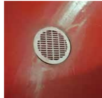
Waste water drain filter.
