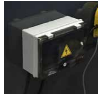
Unloading system stopper box.
