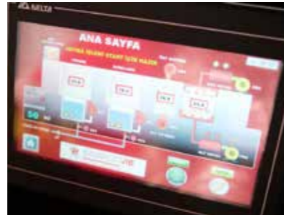
Fully automatic control panel.
