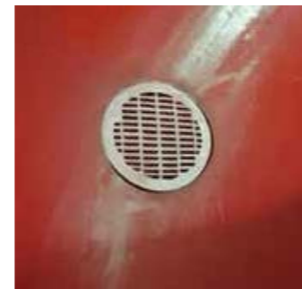
Waste water drain filter.
